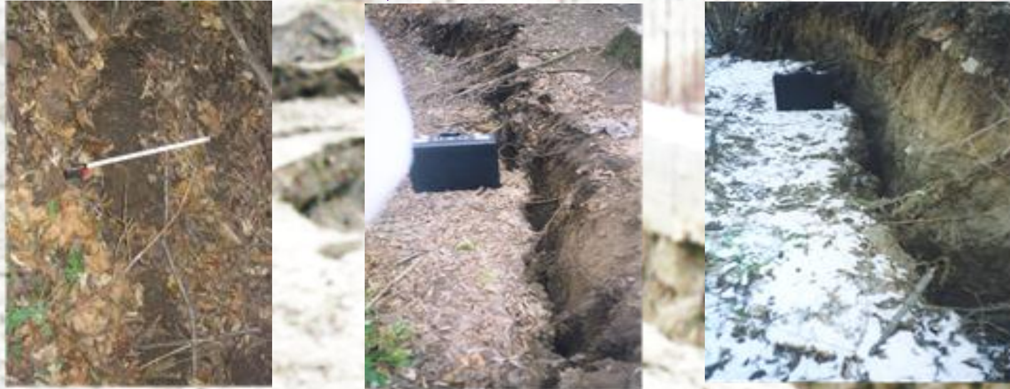
Fig. 2. – Stabbing cracks above the LPS on the slope as of: 1) 28.11.2003; 2) 14.12.2003; 3) 21.12.2003
