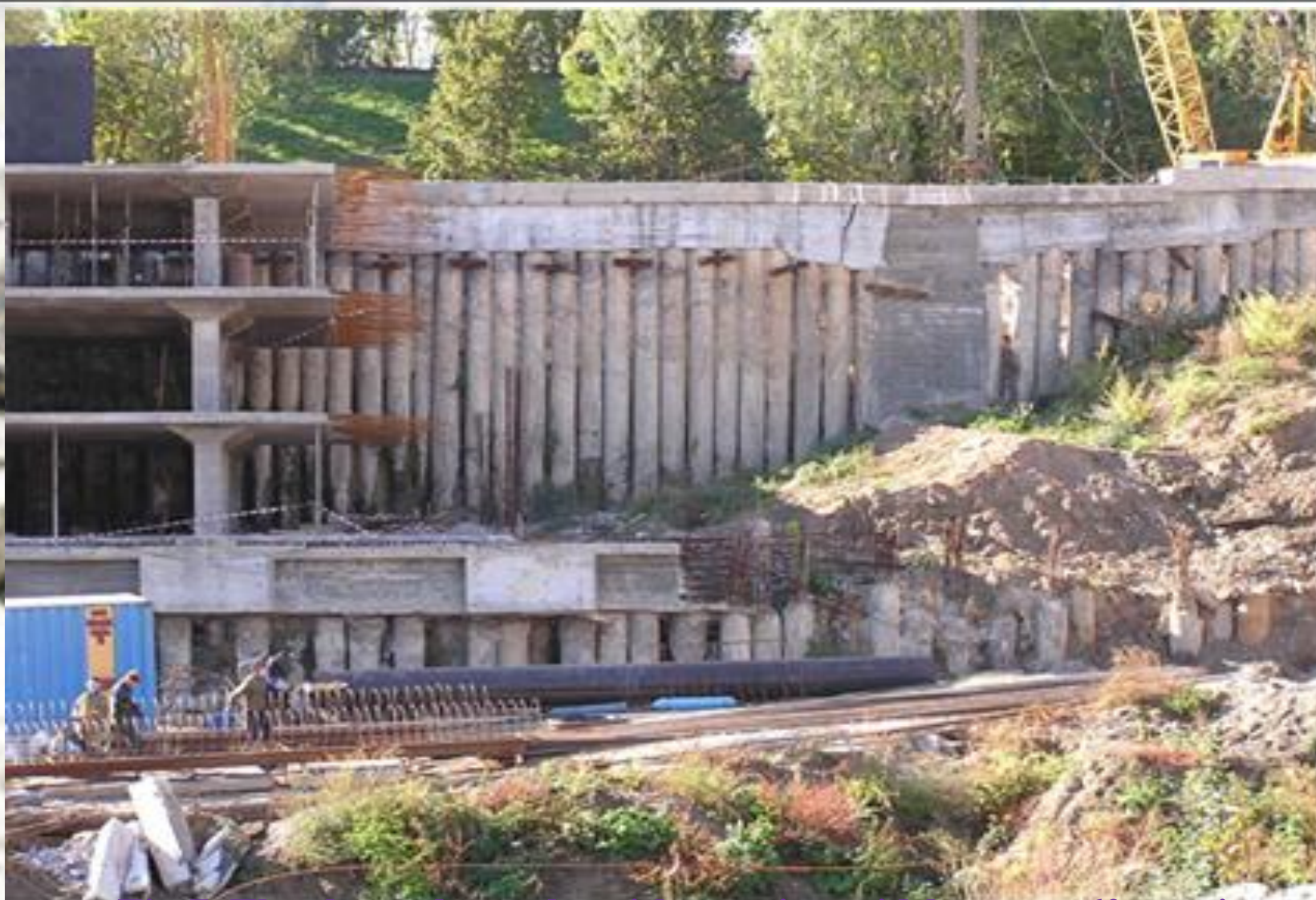
Fig.7. The through cracks with opening widths up to 60 mm in a fence pile ground beam along the Y axis in the 35 ... 37 axes as of
